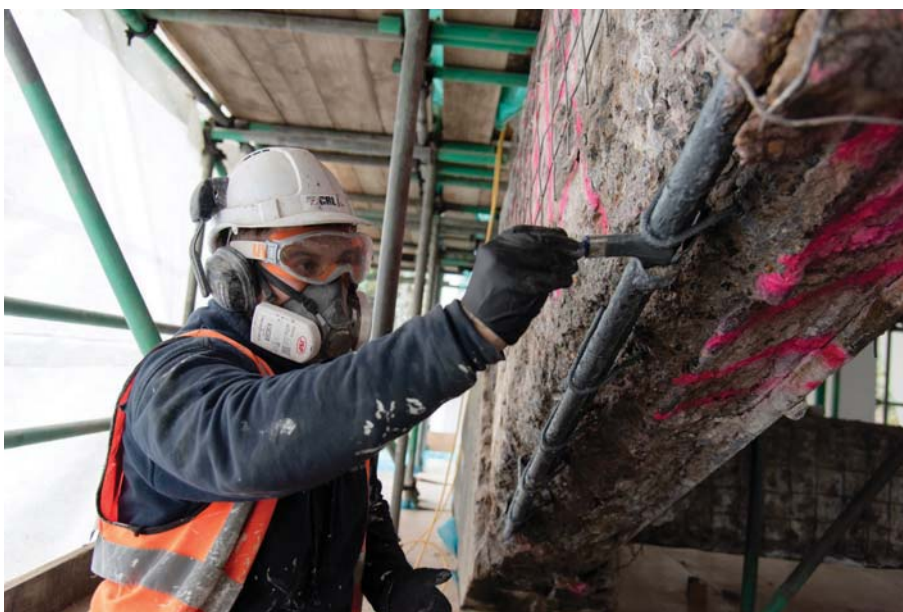
ABOVE MIDDLE: Guniting was removed and new reinforcement fabric fixed to the substrate.
