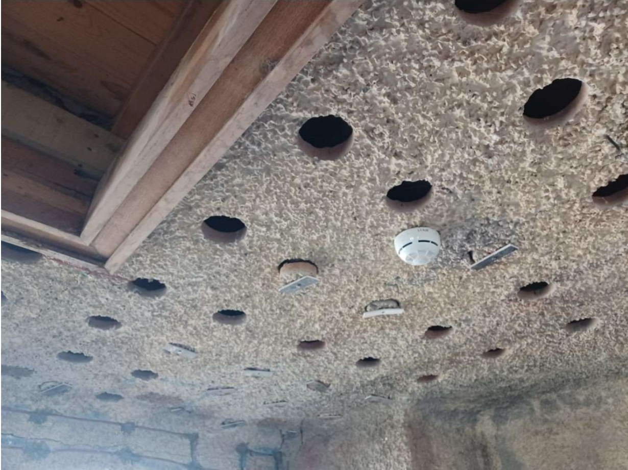
Holes cored through the render and terracotta pots for anode installation © CPT
