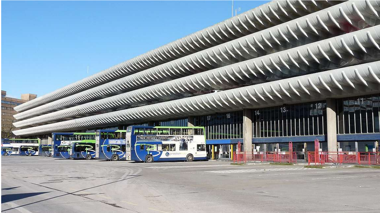
Preston bus station multi-storey car park contains steel at risk of corrosion © CPT
