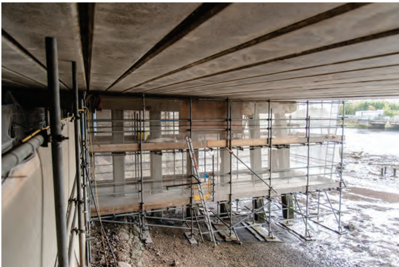
Scaffolding column bent at low tide.
