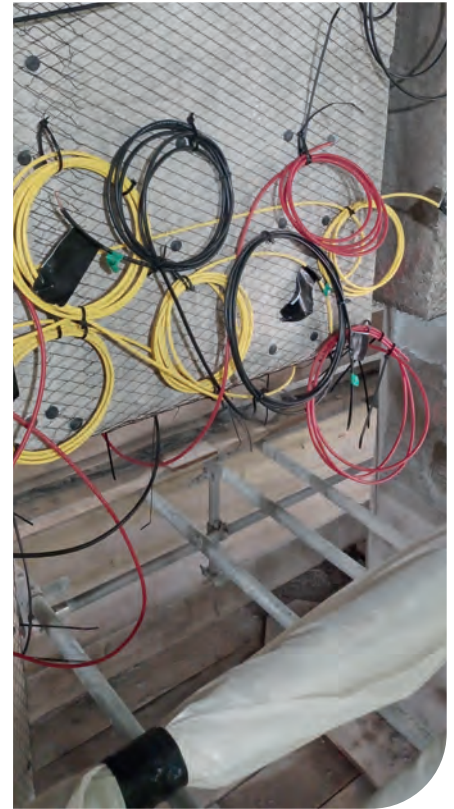
ABOVE: Figure 7 – the impressed current (fabric and overlay) cathodic protection system.
