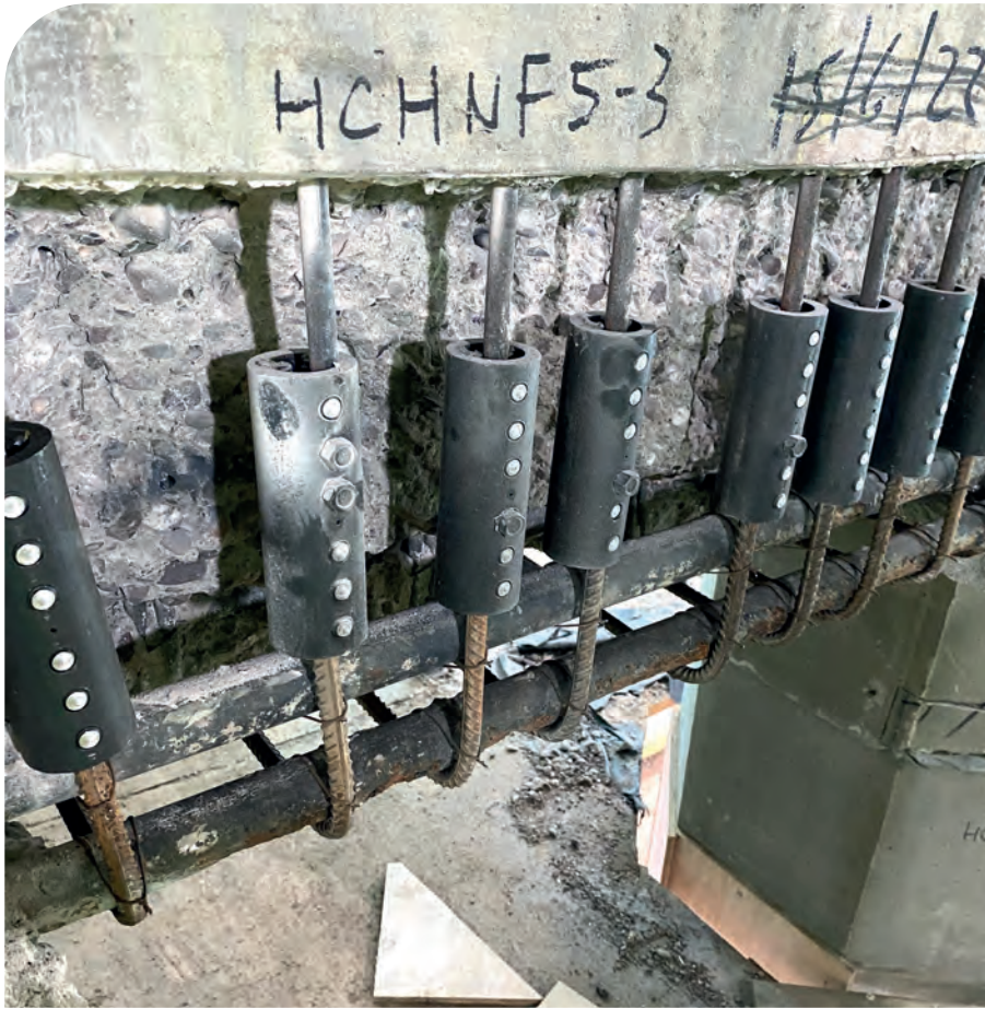
ABOVE: Figure 6 – couplers used to connect the new/replacement reinforcing to the existing.
