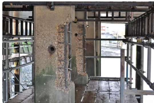
Figure 5 left: Areas of piles where loose, cracked, spalling concrete has been removed with hydro-demolition.
