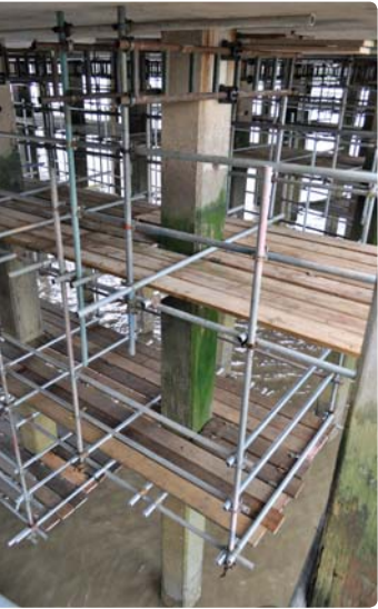
Figure 8 above: Typical access to piles (note the three lifts required to access the full height of the pile).
