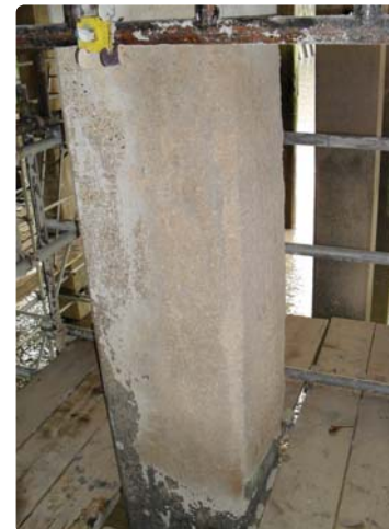
Figure 6 below: Repaired pile showing reinstatement of a patch using Natural Cement's Shotcrete 530 dry spray concrete.
