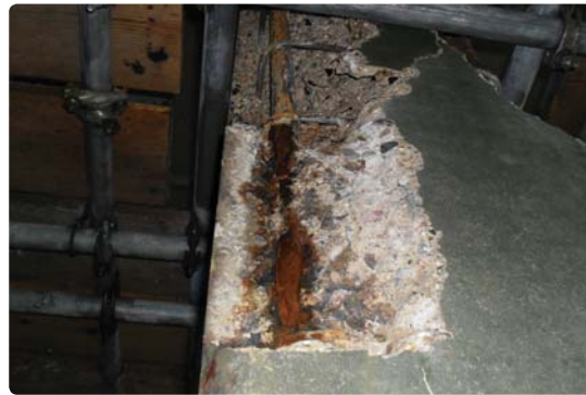
Figure 3 far left: Cracks to pile arrises along vertical reinforcement bars due to the expansive forces caused by the corrosion of the reinforcement.
